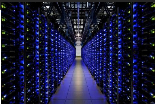
Cloud Data Center
